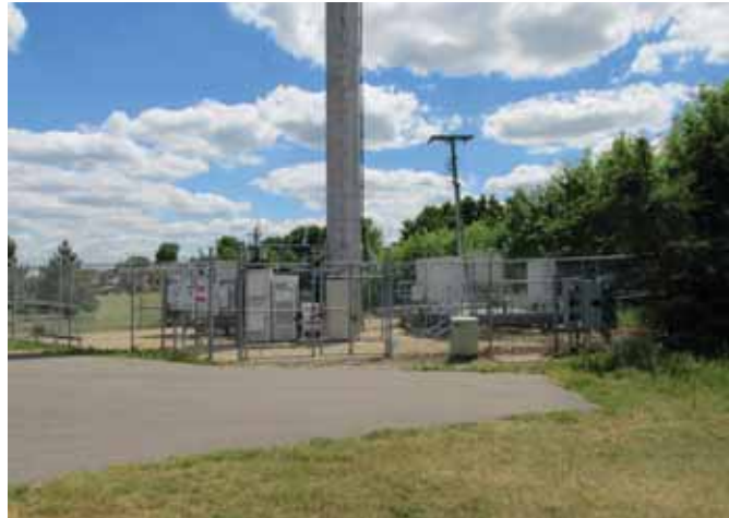
Existing cell tower fence and equipment
